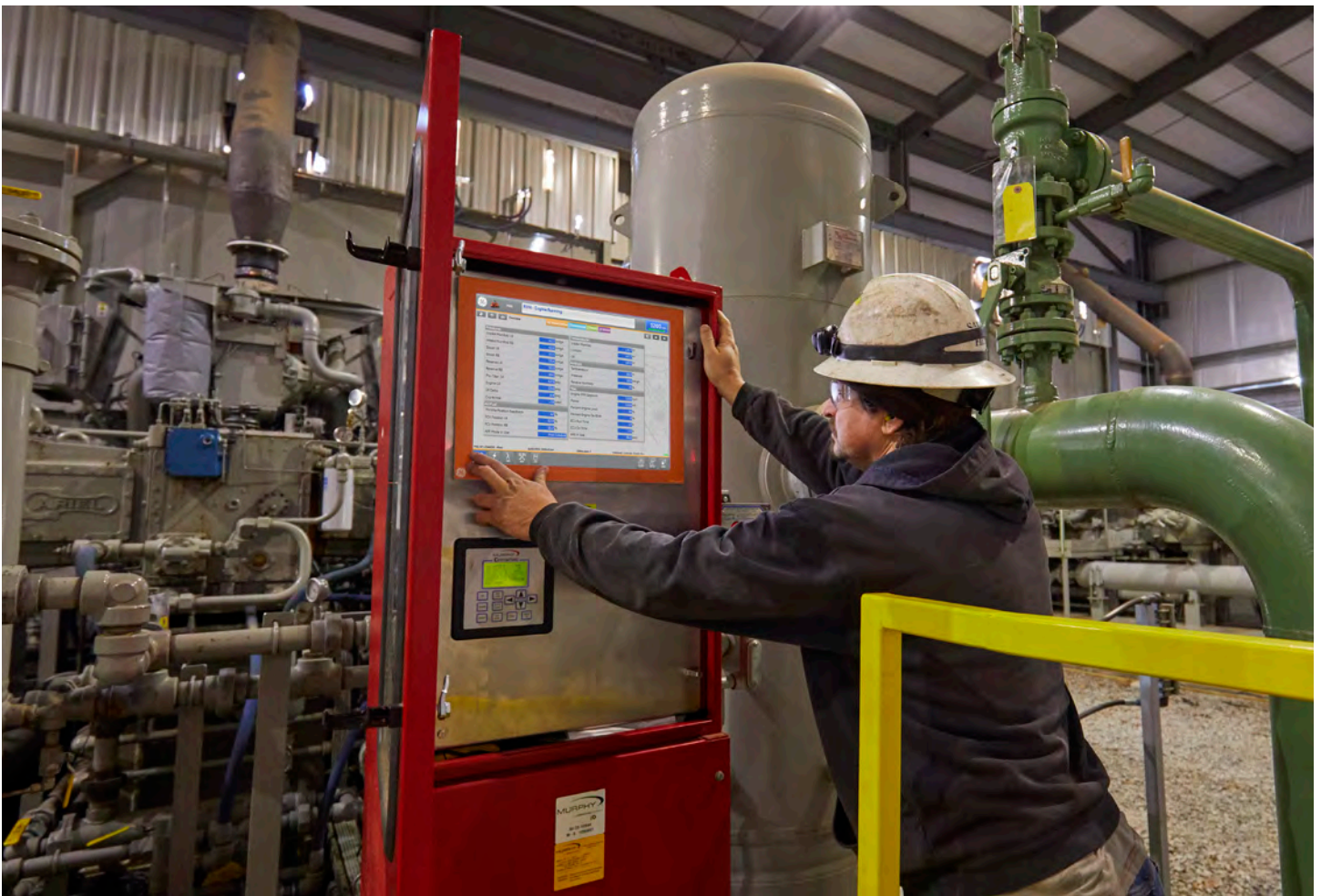
ESM2 HMI display panel operating on a L7044GSI S5 gas compression package
