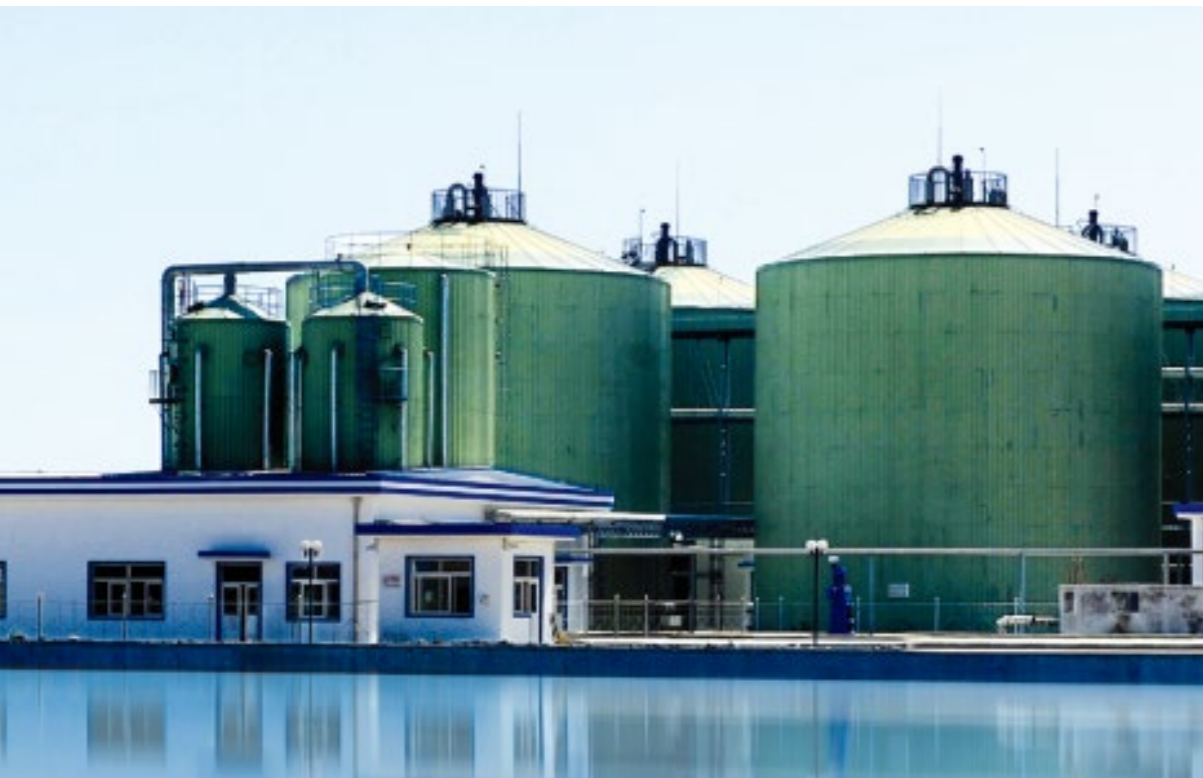
Chicken farm biogas project in Penglai City—Shandong Province, China
